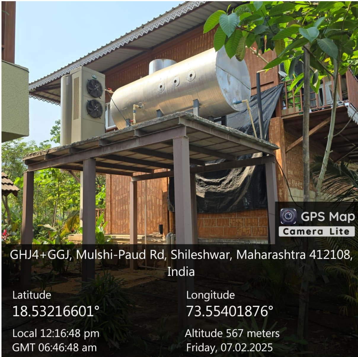
Hot water Generator
