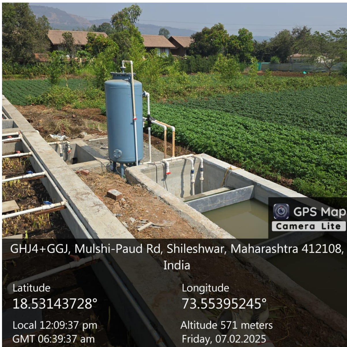
Sewage Treatment Plant (STP) – 30 CMD
